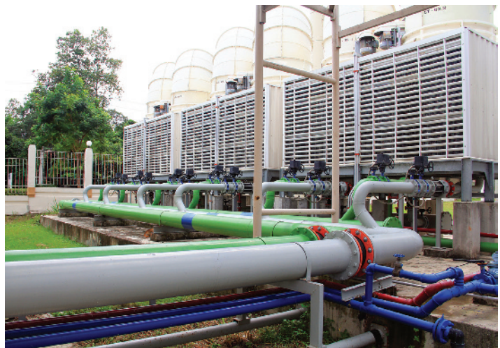
FIGURE 1.1 Complex industrial and commercial fluid piping systems, often unnoticed but critical in our daily lives, require careful design and analysis. The system shown here is required to maintain comfortable temperatures in a commercial building. (Source: Tinnarat Suwanna/123RF)
