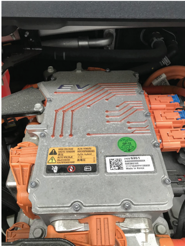
FIGURE 1-2 The orange cables connect to the high power distribution module (HPDM) on the Chevrolet Bolt.
