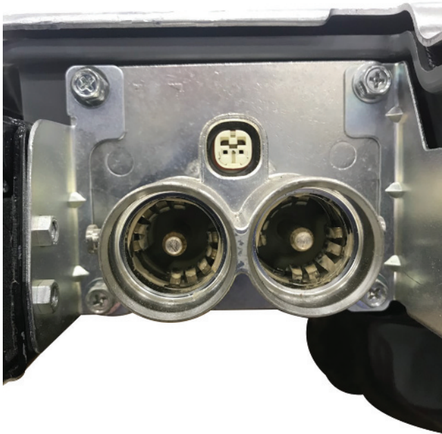
FIGURE 1-19 The small white connector is the local interlock on the HV connection to the battery.
