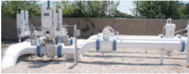
FIGURE 1-4 Natural gas pig insertion and recovery station.
